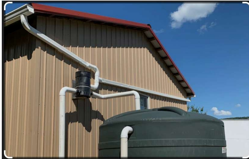
Figure 13.1: Rainwater Storage Unit
